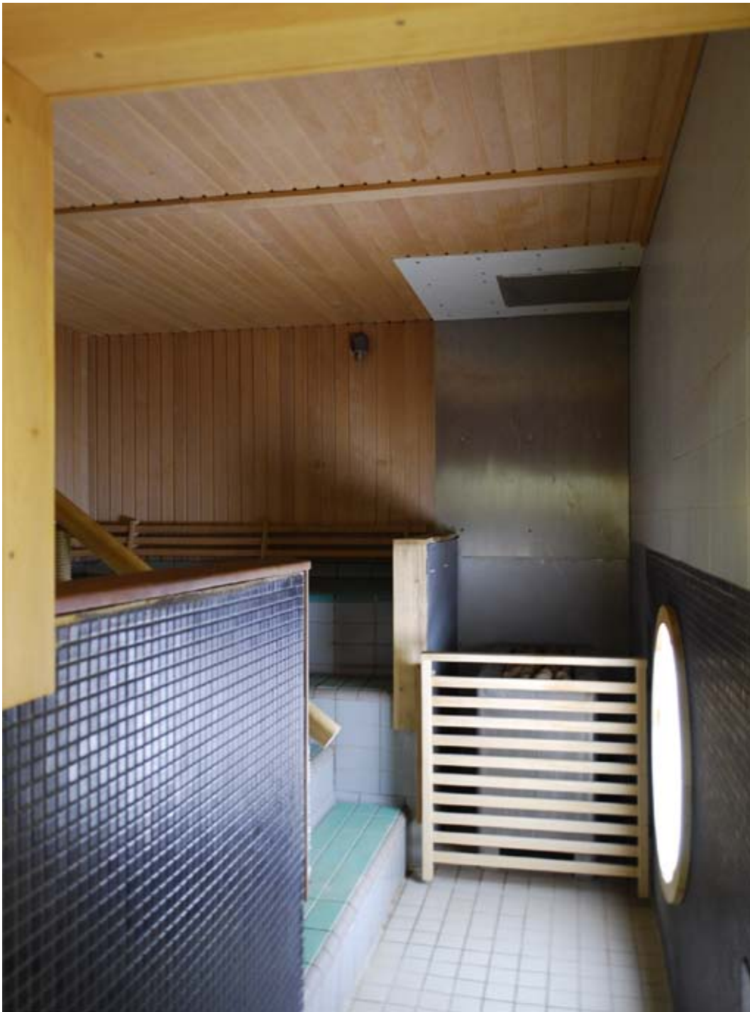
Figure 9 & 10. Swimming hall partition walls (multiple wall sections)
